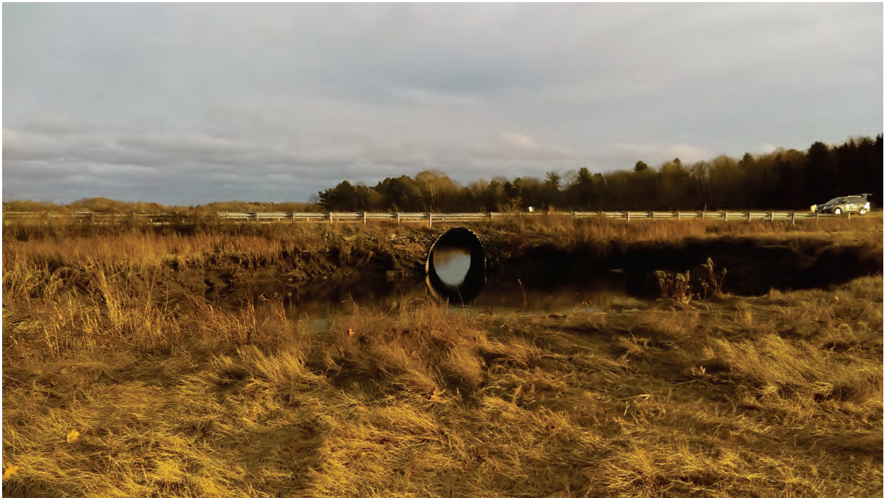
Existing Aluminum Culvert Crossing at Sawyer Road (Photo Credit: Wells National Estuarine Research Reserve)
