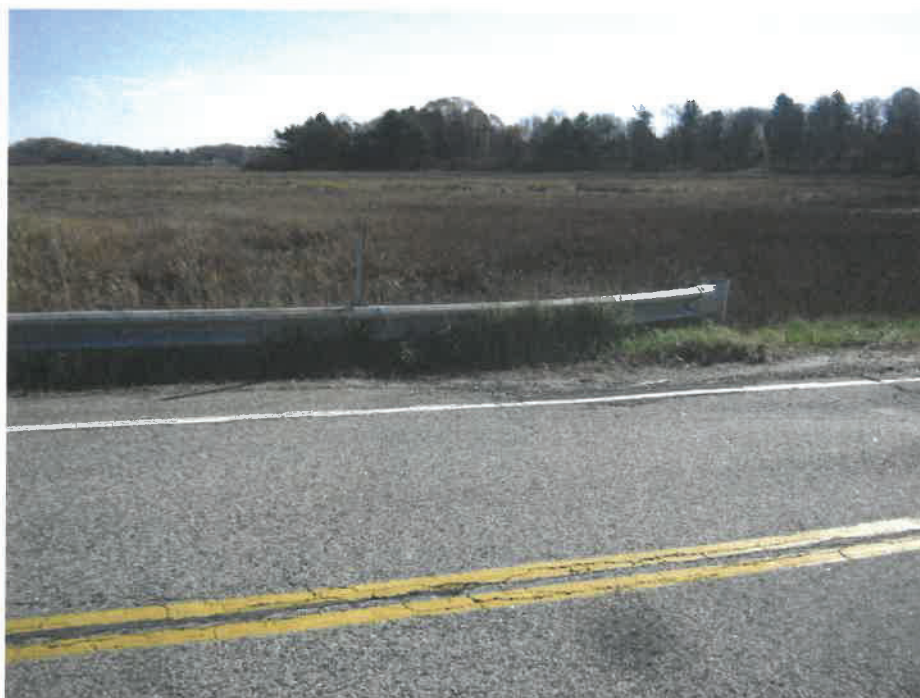
PHOTO 6 Description View showing low approach rail
