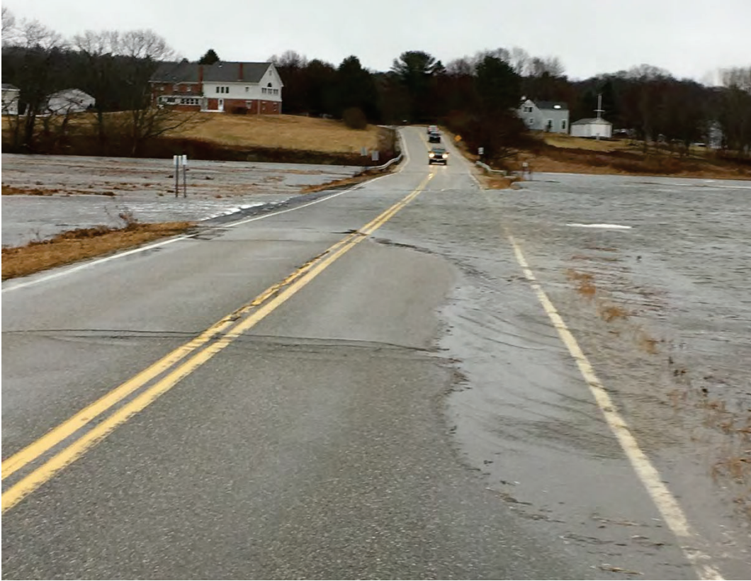
Sawyer Road Crossing Overtopping During High Tide on 3/2/2018 (Photo Credit Town of Cape Elizabeth)
